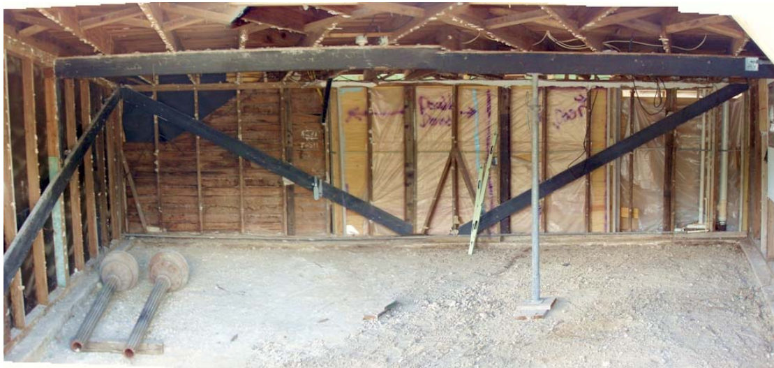
The ground floor stripped of all the gypsum board. Note the plywood on the back wall where the new doors will go and also the two lamp posts laying on the ground.
