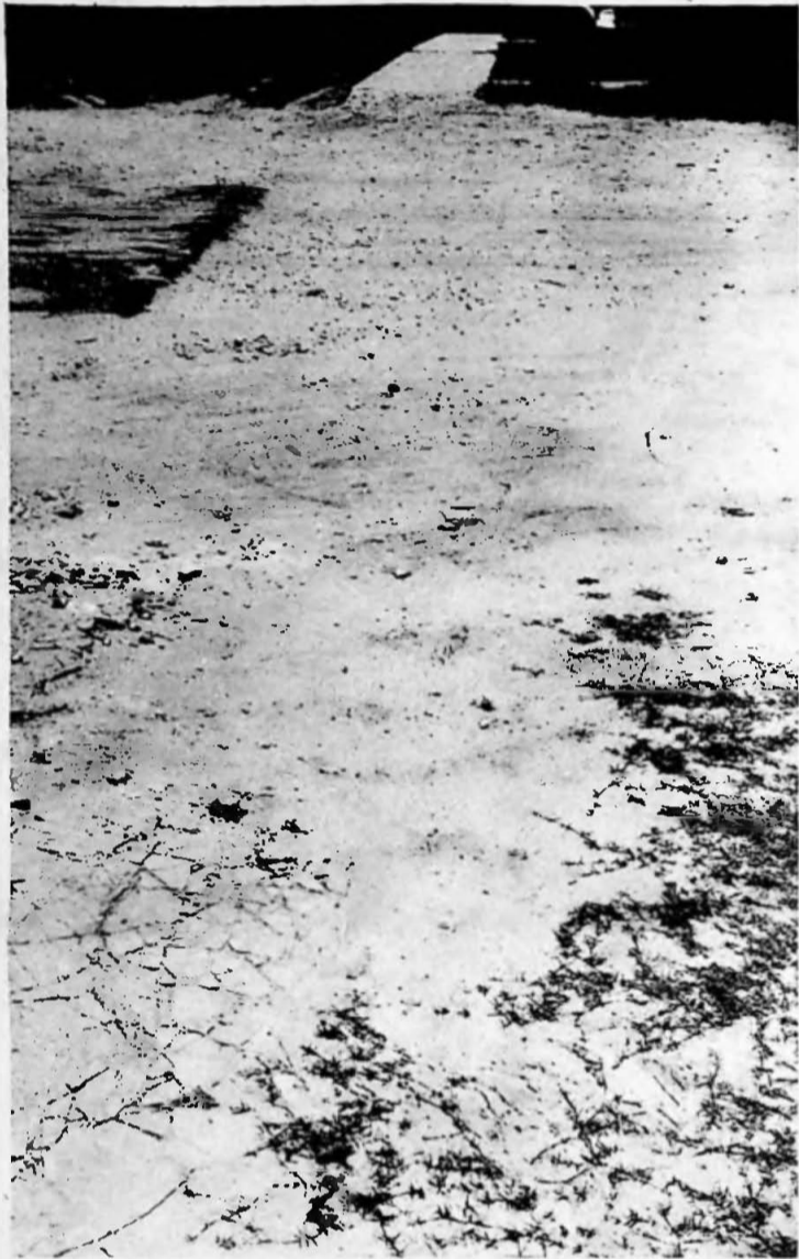
ANKIE TURNING ROCKS AND PIECES OF CONCRETE UP TO THE SIZE OF GOLF BALLS LITTER THE SPACE WHERE A SIDEWALK WAS BEFORE ROAD CONTRACTOR'S HEAVY MACHINERY DEMOLISHED IT. LOCATION IS IMMEDIATELY SOUTH OF MILLER HARDWARE ON WILTON DRIVE.
