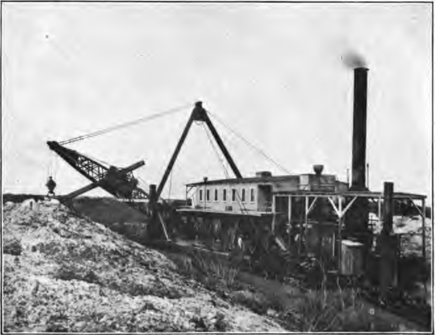
FIG. 1.—STATE DREDGE OKEECHOBEE CUTTING THROUGH THE ROCK RIM ON THE EAST SIDE OF THE EVERGLADES.
