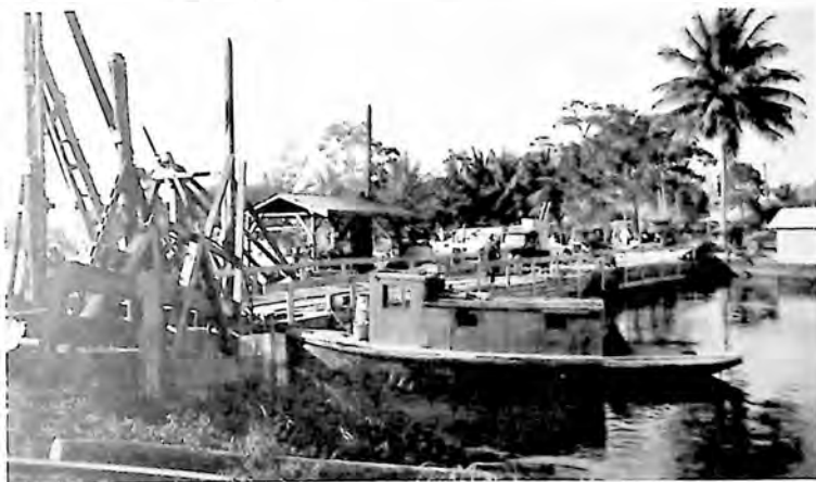
Below: Pontoon bridge used during construction of Broward's first lift bridge over Andrews Avenue
